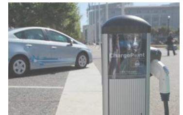
EV Charging Stations
