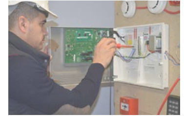
Fire Safety Alert Systems
